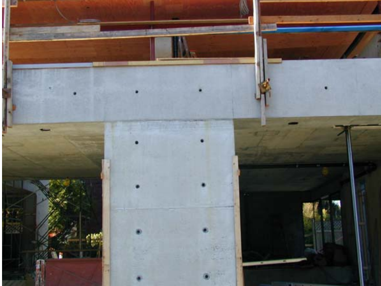
Figure B-3: Close-up of Form Fresh Finish, Wall and Slab Edge Cold Joint
